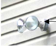
Unshielded Floods Aimed Out/Up
